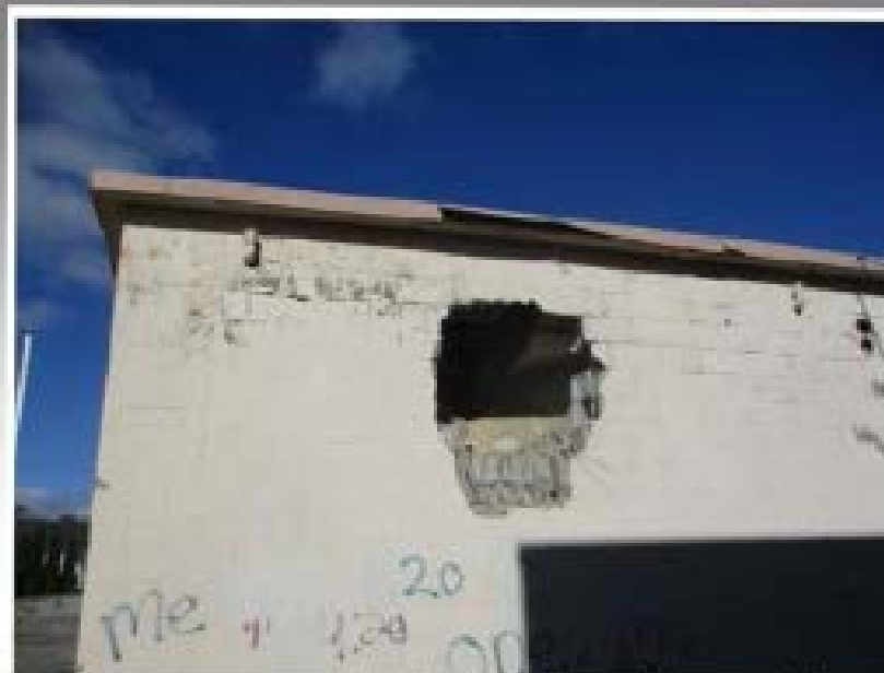
Photo 4 (6-27-17): Vermiculite insulation within AST bunker (sample set 62); ACM (Tremolite) found to be present.
