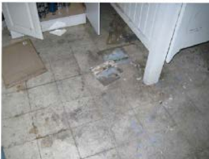
Photo 10 (6-27-17): ACM 9-inch floor tiles (sample set 09) located in bathroom within Site Building Room 22.
