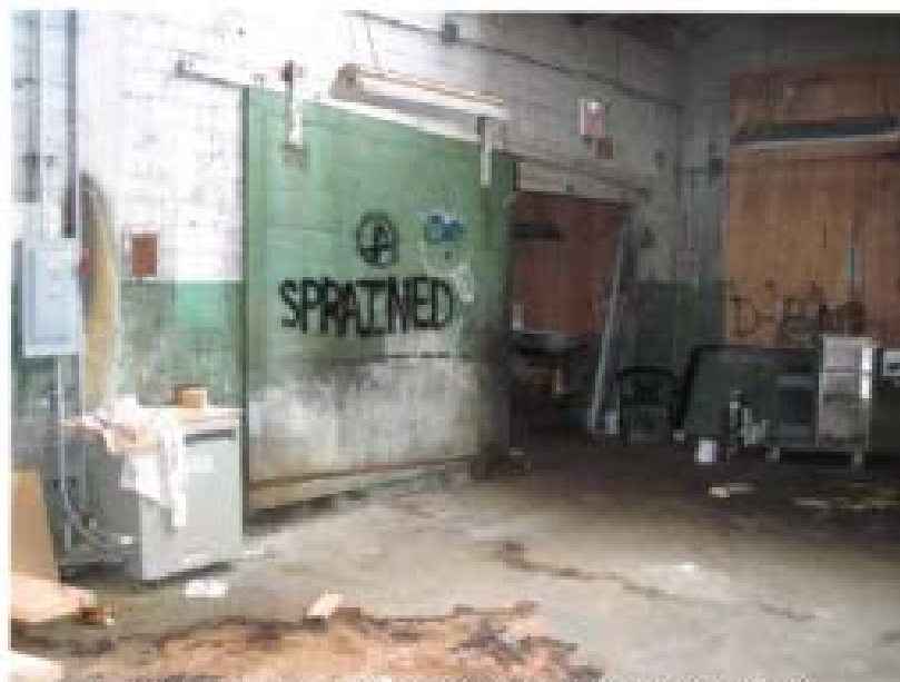
Photo 14 (6-27-17): One of several fire doors observed throughout the Site Building interior (P.A.C.).
