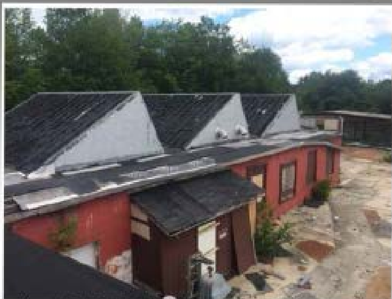
Photo 17 (6-27-17): View of 'sawtooth' skylight area with ACM roofing applied to the shallow slope, and ACM flashings.
