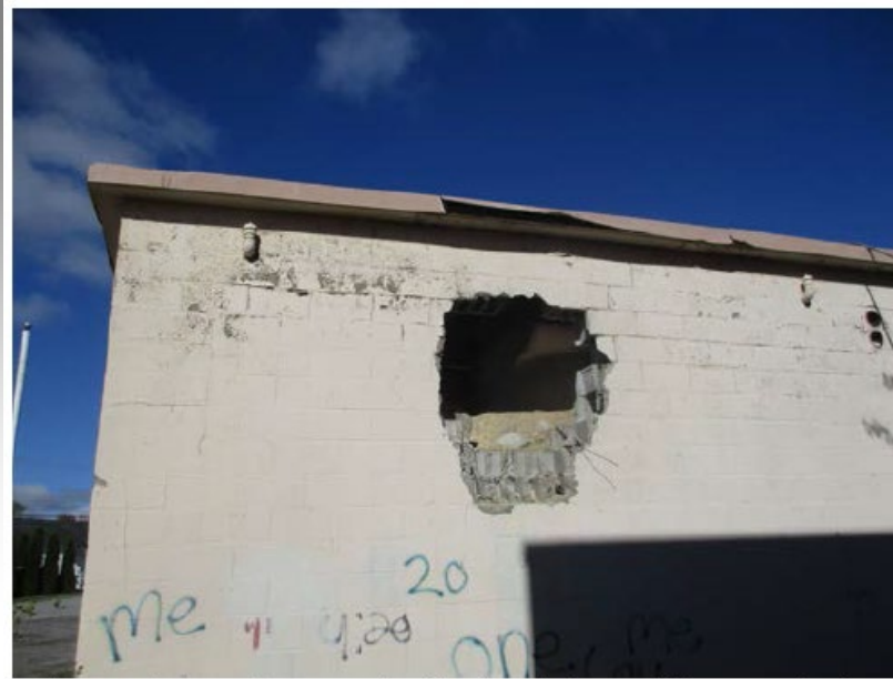
Photo 4 (6-27-17): Vermiculite insulation within AST bunker (sample set 62); ACM (Tremolite) found to be present.
