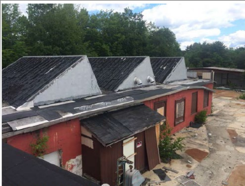
Photo 17 (6-27-17): View of “saw tooth” skylight area with ACM roofing applied to the shallow slope, and ACM flashings.
