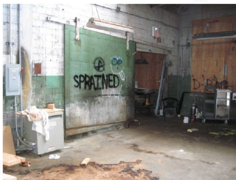
Photo 14 (6-27-17): One of several fire doors observed throughout the Site Building interior (PACM).
